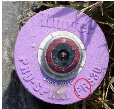
Figure 1 Pressure regulating irrigation is identified with a PR” and can be visually inspected as pictured
