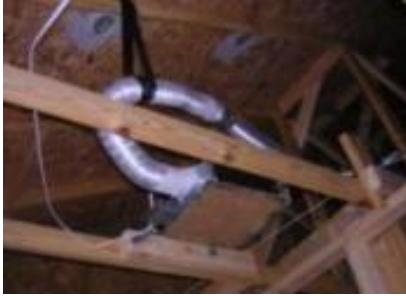
Figure 1 Poor installation (U bend)
